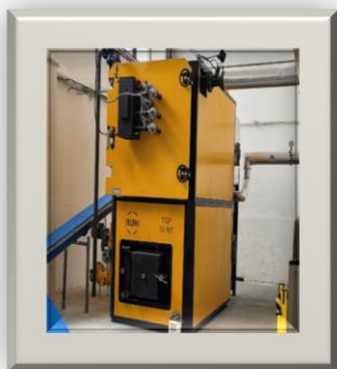
New wood chip boiler
