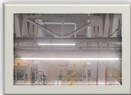
New LED lights
